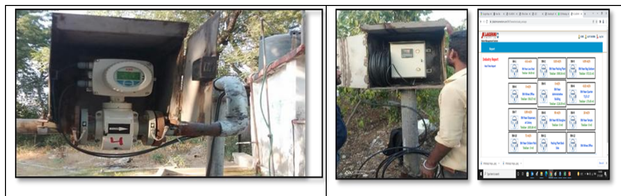
A Visual of Digital Water Flow Meter, Digital Water Level Recorder along with telemetry system.
