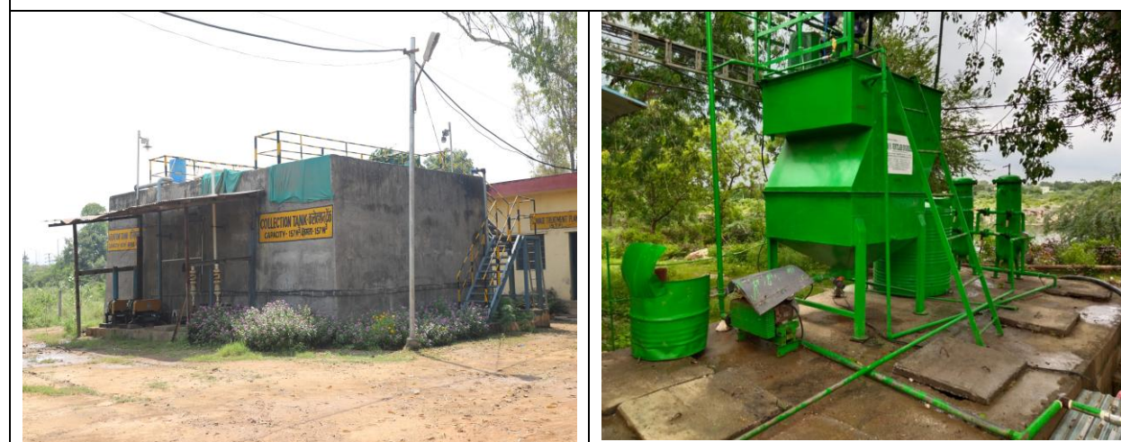
Sewage Treatment Plant
